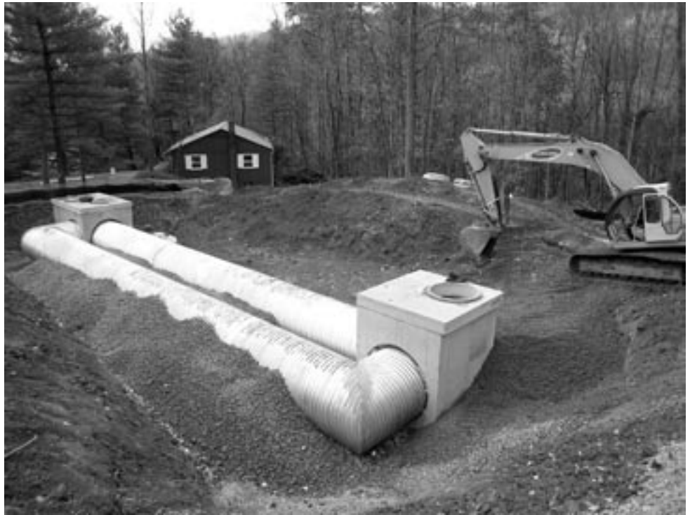
This system, now buried under a new parking lot, provides temporary storm water storage to buffer the impact of runoff on local streams and ponds.
