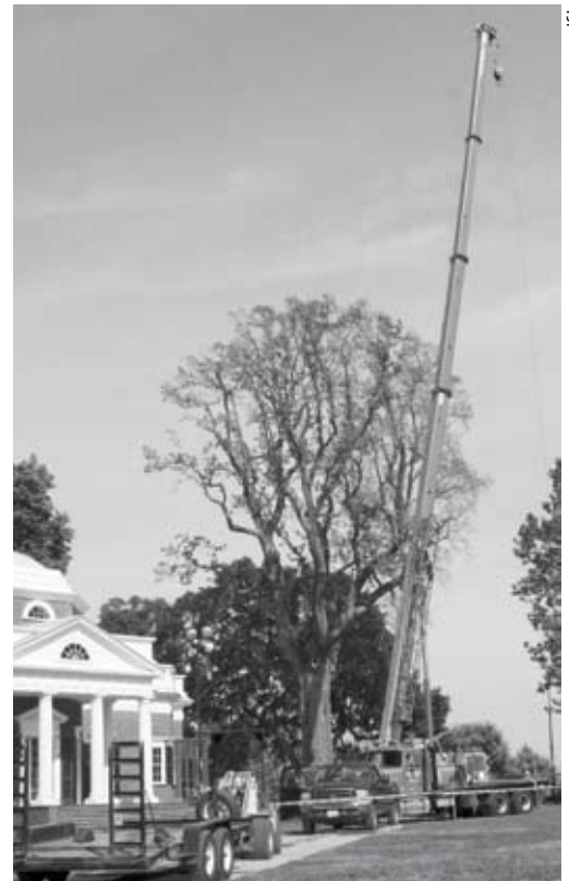
A 90-ton crane was employed in removing the tulip poplar from the side of the house.
