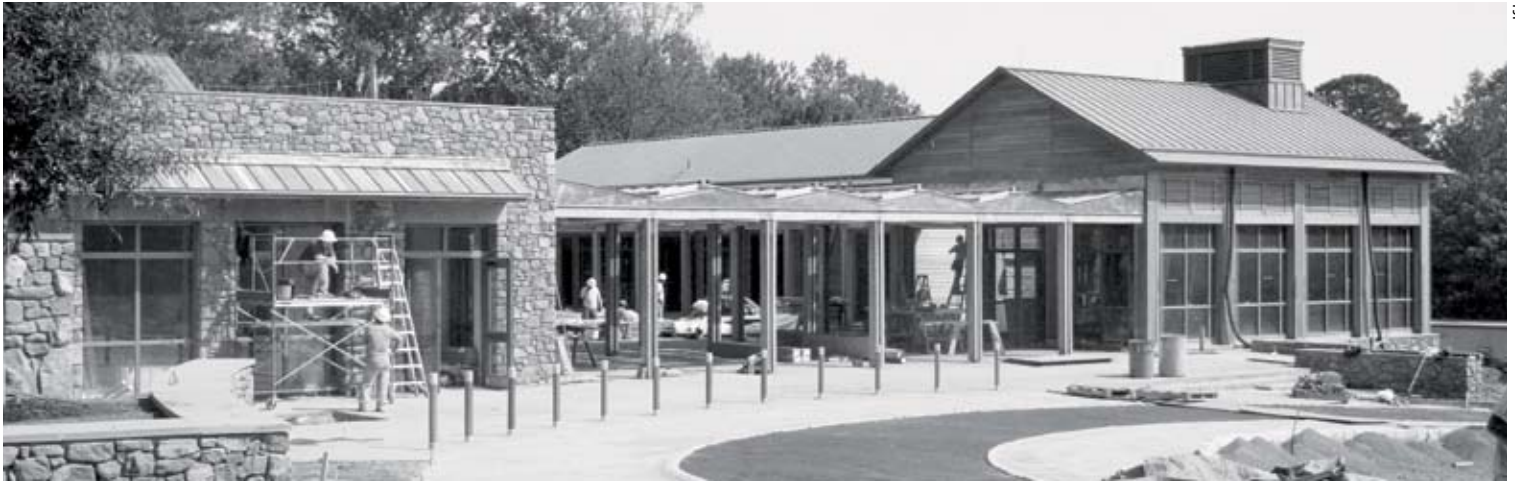
The west front of the Thomas Jefferson Visitor Center and Smith Education Center during the latter stages of construction. On the left is the Museum Shop; the Welcome Pavilion is to the right.
